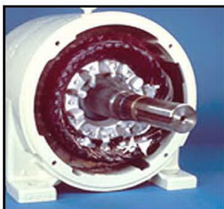
Damage Caused by Locked Rotor
